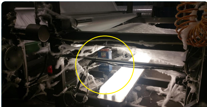
IntelliSENS speed and length sensor installed on Monadnock's non-woven lines
