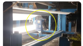
IntelliSENS speed and length sensor measuring on-line at Monadnock
